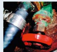
Many used boats have gate valves. This one is terminally corroded
